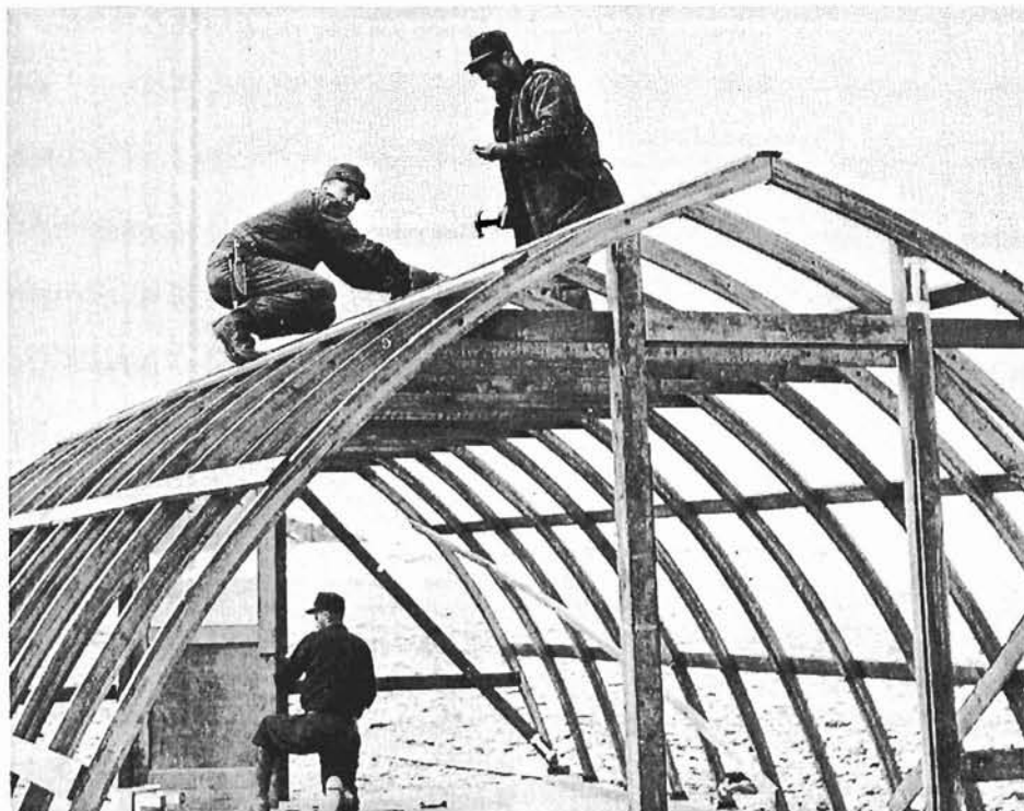
Flown from the Labrador by helicopter over miles of ice-clogged sea, an Atwell shelter to house personnel operating electronic position indicator equipment is assembled by Able Seaman Burton Reid and Walton Chipman and (below) CPO Riley Mombourquette. (LAB -930)
